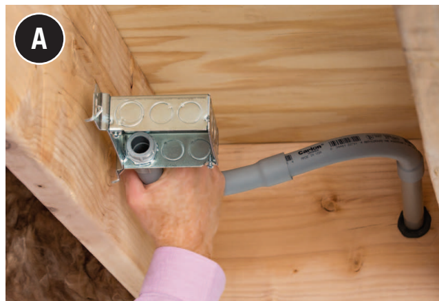
Cable from a new breaker in the main service panel runs to an electrical junction box near the point where rigid conduit runs to the exterior, usually through a hole drilled into the rim joist.
