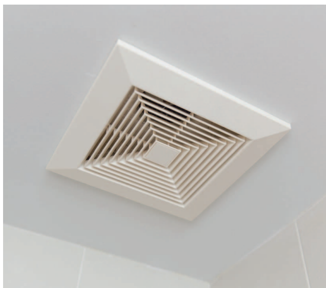
A ceiling vent fan , or one mounted at the top of a wall or at floor level, provides air movement and exhausts undesirable air impurities.
